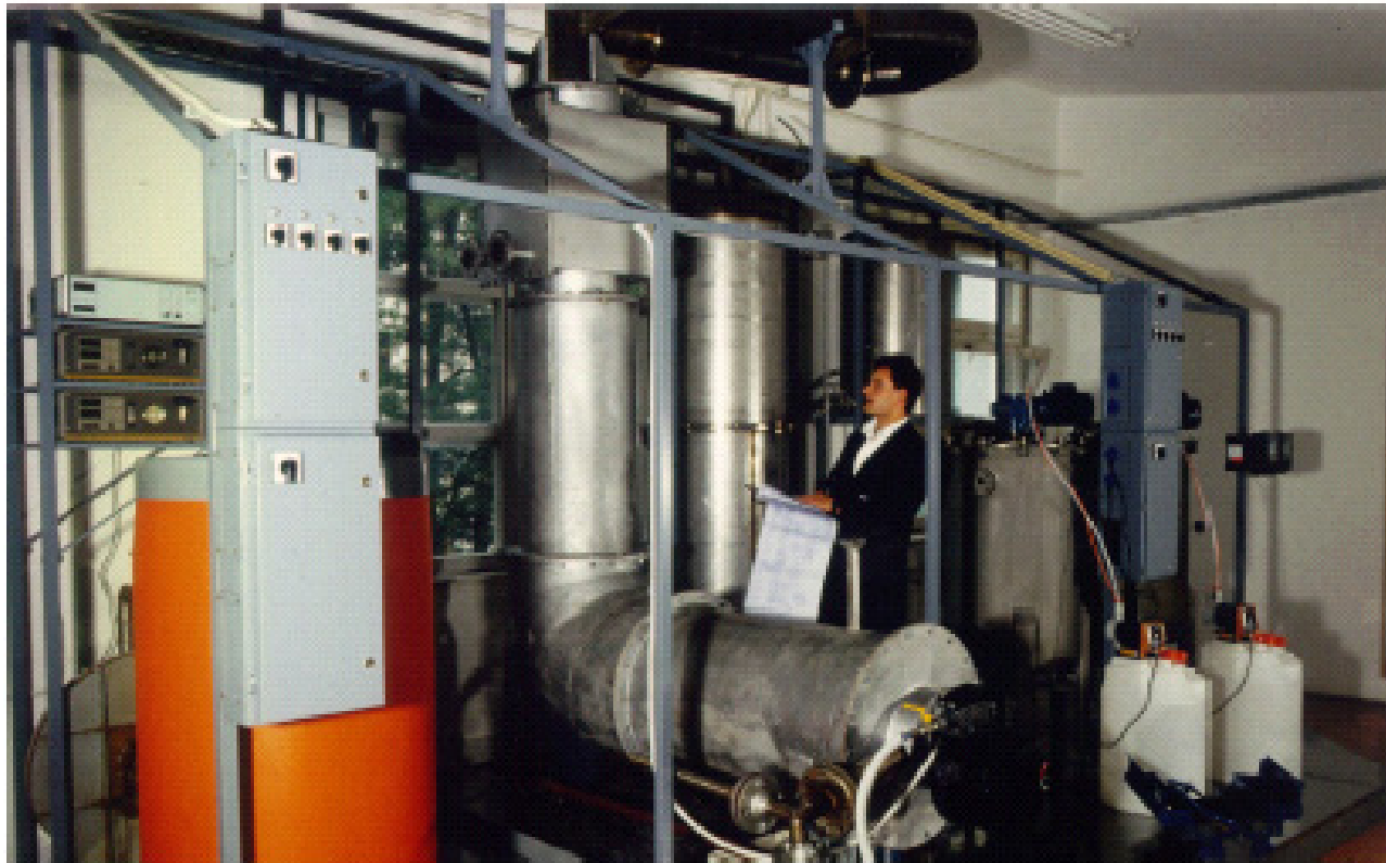
Pilot installation at Jozef Stefan Institute, Slovenia
